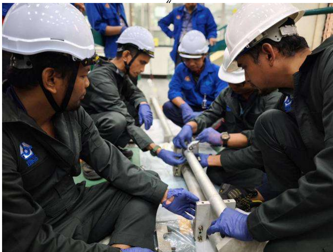
Photo 6.2: Installation of Nuclear Fuel Integrity Inspection Equipment
