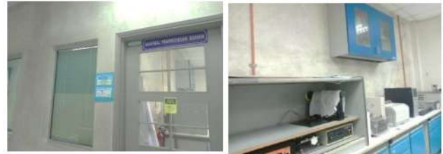
Figure 1: Wall with fungus existence in Block 34.
