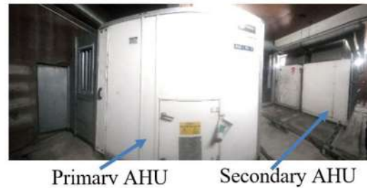
Figure 3: Arrangement of air damper, primary AHU and secondary AHU in AHU Room Block 19.
