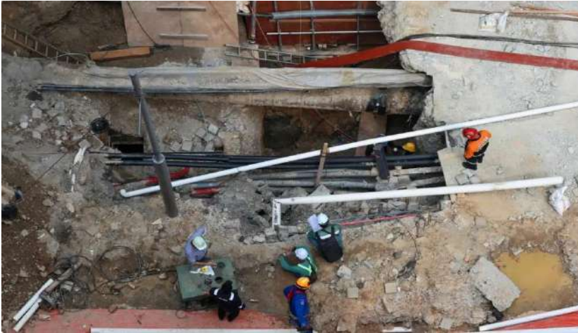
A view of the search efforts yesterday at the site in Jalan Masjid India where a woman fell into a sinkhole on Friday, Aug 23.
